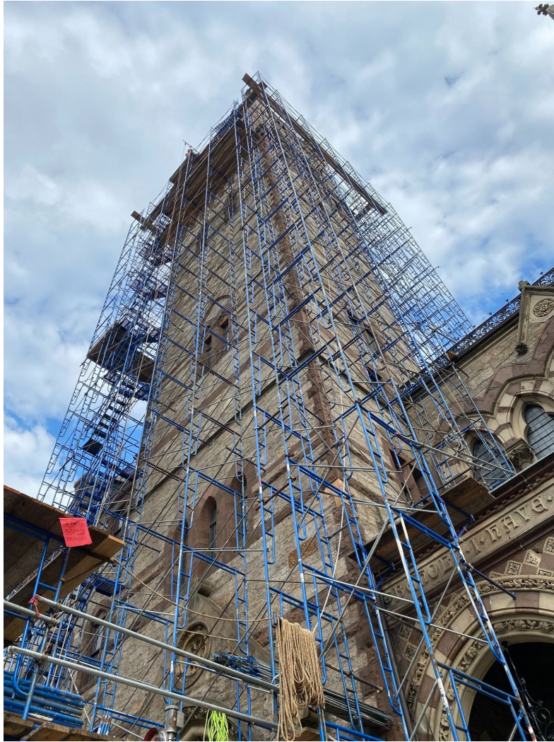
Scaffolding work continues on Old South's Tower. Photo by Nancy S. Taylor
